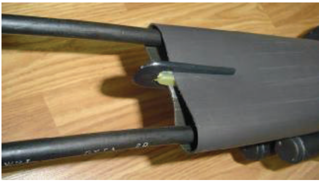
(14) Use a branch fork: when heating the oval entry port, fork the heat-shrinkable tube to separate the two cables and heat-shrink it --follow the steps above.
