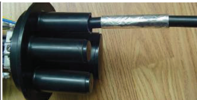
(12) wrap and even the heat-shrink part with aluminum paper to avoid overheating caused by high temperature burner.
