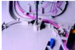
Fiber Fan-Out (Pre-Terminated Splitters)
